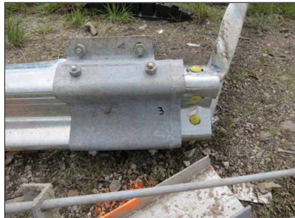
Figure 5: End of guardrail panel 2, beginning of panel 3. Note unsheared splice bolts
