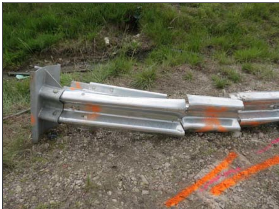
Figure 4: Guardrail panels 1 and 2, cut by rescue personnel
