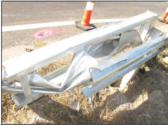
Figure 10. Northwest-facing view of the end terminal and deformed W-beam.
