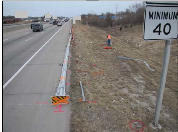
Figure 1. View east to the damaged guardrail.
