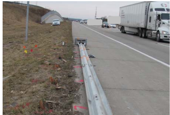
Figure 9. Fractured posts 1 - 7, view west.
