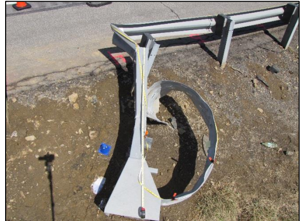
Figure 9. Overhead view of the location of the displaced end terminal.
