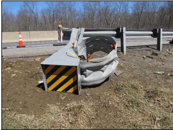
Figure 8. Image depicting the impacted end terminal and the extruded W-beam.
