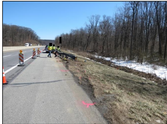
Figure 3. Eastbound view of the shoulder, roadside and struck SKT guardrail end treatment.
