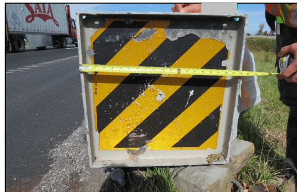
Figure 7. The damaged end terminal.
