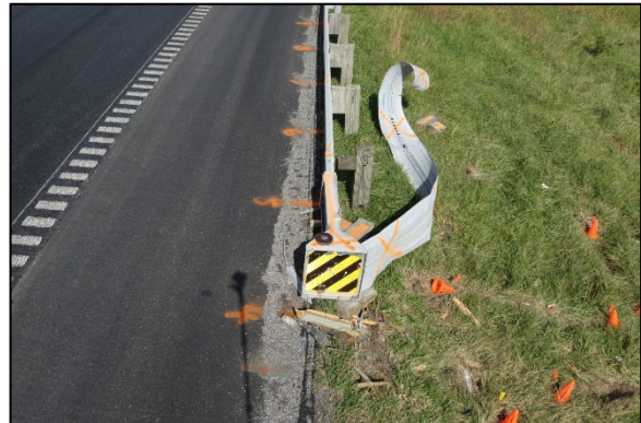
Figure 1. The damaged end terminal and guardrail.
