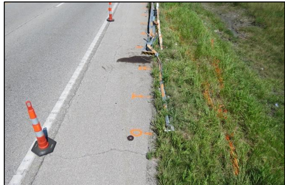
Figure 1. Overhead view of the damaged end terminal and guardrail, view north.
