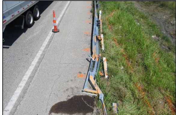
Figure 8. Damaged posts and guardrail, view north.
