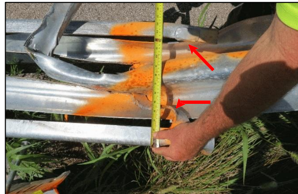
Figure 9. Sliced section of the guardrail and fractured cross-brace (arrows) at the entrance to the feeder channel.
