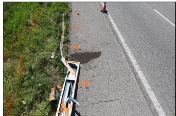
Figure 7. Extruded guardrail from the end terminal, view south.
