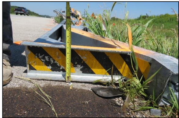
Figure 4. The damaged end terminal, view north.
