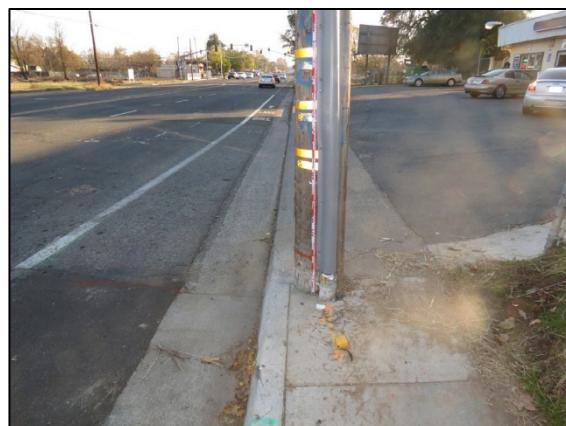
Figure 4. Struck utility pole, looking south.
