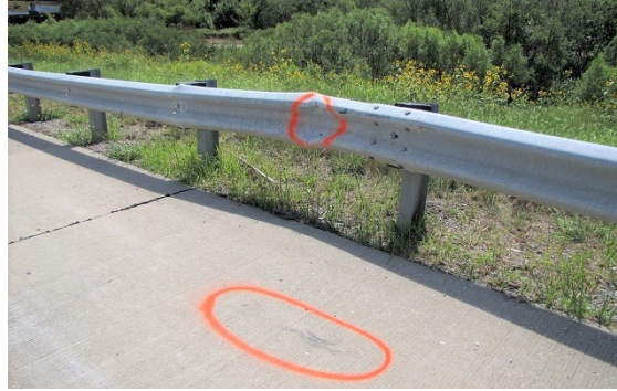
Figure 6. Second guardrail impact, right shoulder
