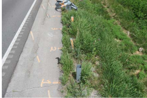
Figure 4. North-facing overhead view of the damaged guardrail. (Post 1 reinserted to pre-crash location)
