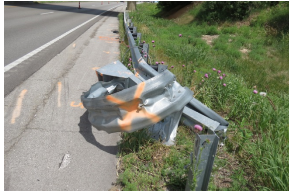
Figure 6. Northerly view, extruded and kinked guardrail.
