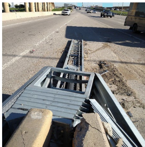
Figure 5. North-facing lookback view of the deformed attenuator
