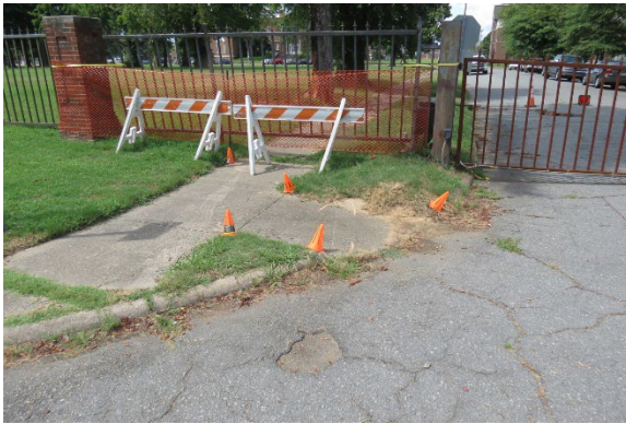
Figure 4. North view, roadway departure and impact with fence (replaced since crash)
