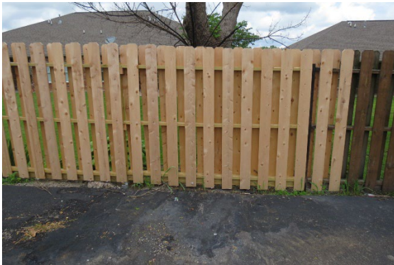
Figure 4. North view, impact with wooden fence (replaced)
