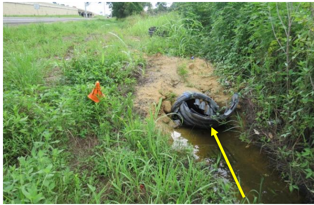
Figure 4. Northeast view, plastic culvert pipe contacted by the front lower plane of the Ford
