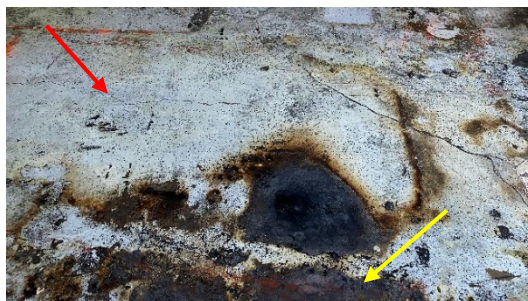
Figure 6. Fire damage to the garage floor under the left side of the vehicle
