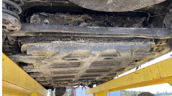
Figure 9. Rear view looking forward of the 60 kWh Li-ion battery pack in the involved 2019 Chevrolet Bolt
