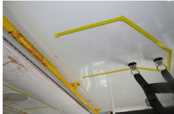
Figure 9. Closeup of contact to ceiling rail and blood mist/splatter on ceiling
