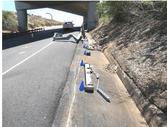
Figure 6. Guardrail impact damage looking south, Post 1 in the foreground
