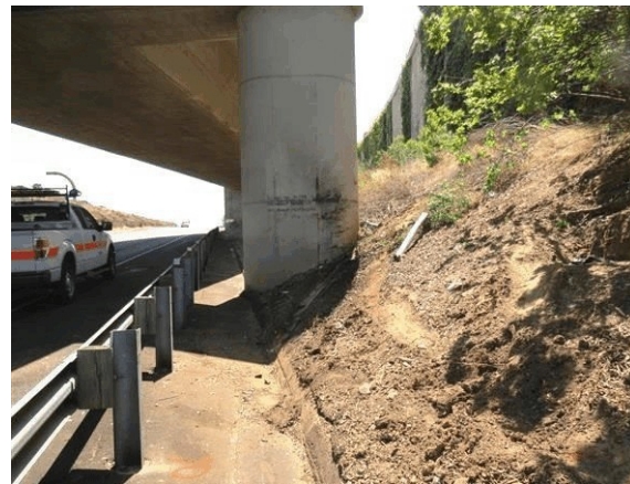
Figure 5. Struck overpass pier, looking south on field side of guardrail
