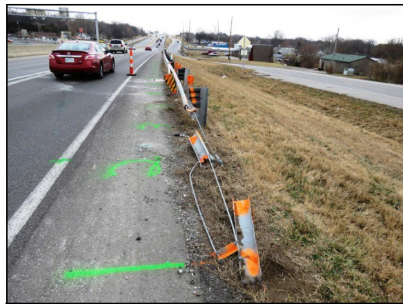
Figure 4: East-looking image depicting the crash site and the X-Lite guardrail end terminal damage.
