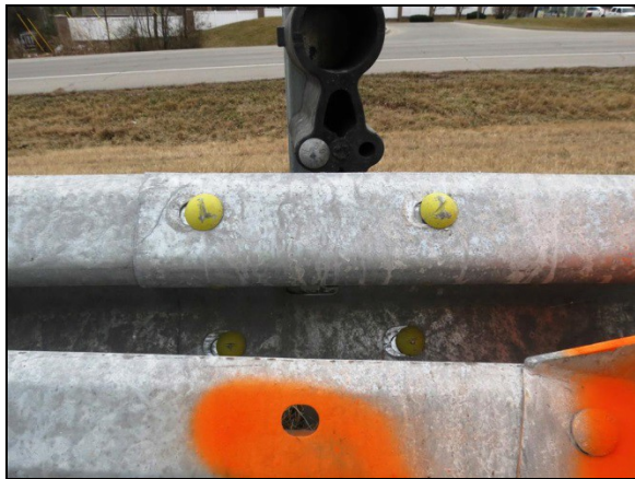
Figure 6: South-looking image of the displaced Panel-1 at Post-5 and the shear bolt connection between Panel 2 and 3.
