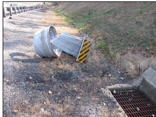
Figure 5: East-looking image depicting the final rest position of the displaced end terminal and extruded rail.
