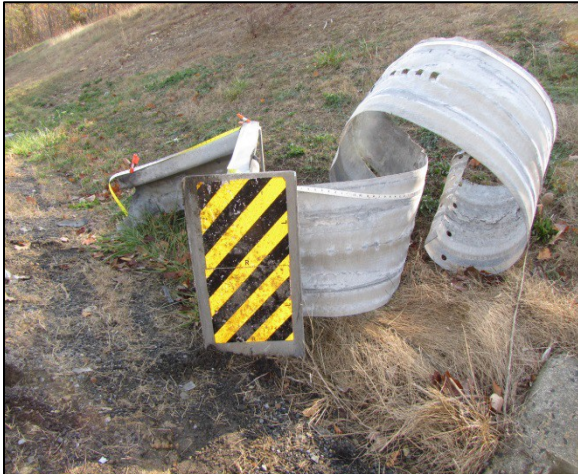
Figure 10: Southeast-facing image depicting the ET-Plus 10 cm (4 in) end terminal and the extruded guardrail.
