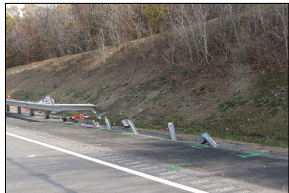
Figure 9: Oblique view of the crash site looking to the southeast.
