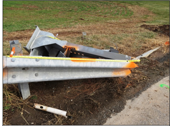
Figure 8: Southeast-facing view of the damaged ET-PLUS end treatment.
