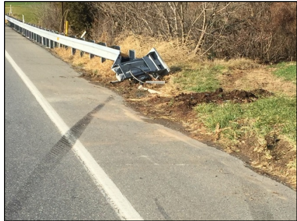
Figure 1: North-facing view of the damaged ET-Plus guardrail end treatment.
