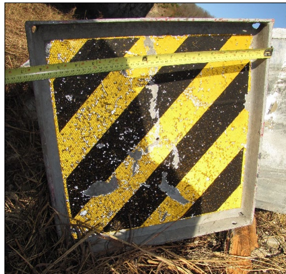
Figure 6: The damaged ET-2000, tape measure in feet and tenths of feet and centimeters
