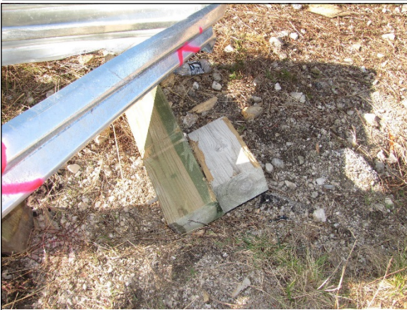
Figure 9: Damaged post 4, view west to field side,
