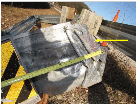
Figure 7: Extruded guardrail from the ET-2000; arrows shows red paint from contact the Toyota's left front door
