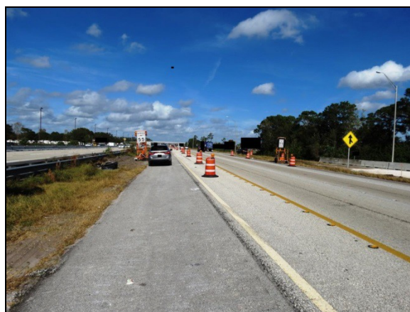
Figure 2: Northbound trajectory view of the crash site at the time of the SCI inspection.
