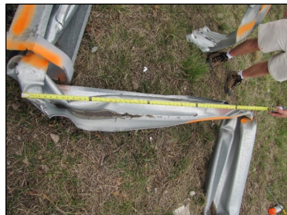
Figure 8: Kink in guardrail at entrance chute to end terminal
