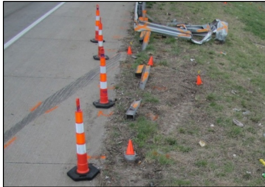
Figure 10: Guardrail separated from posts 1 - 5, view west
