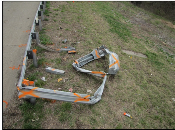
Figure 1: The damaged SKT and guardrail, view west
