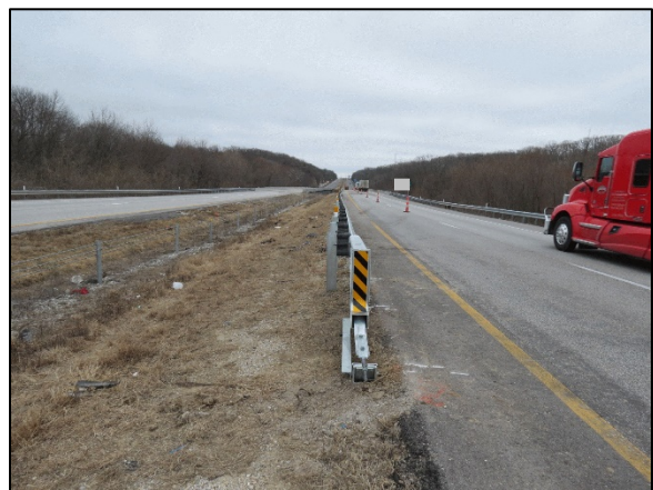
Figure 4: Area of impact with the guardrail, which had been replaced by a Soft Stop system, view east
