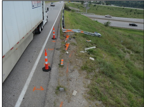
Figure 1: The damaged SKT and guardrail, view south
