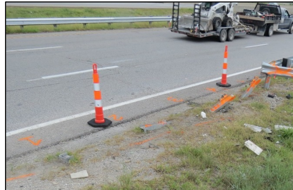
Figure 8: Damaged posts 1 - 5, view southeast
