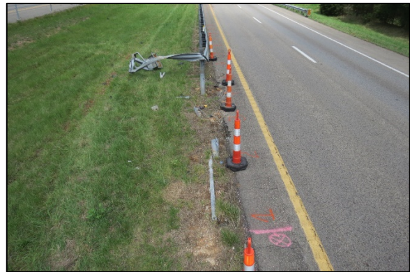
Figure 1: The damaged guardrail and End terminal
