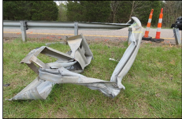
Figure 8: Kinks in the guardrail
