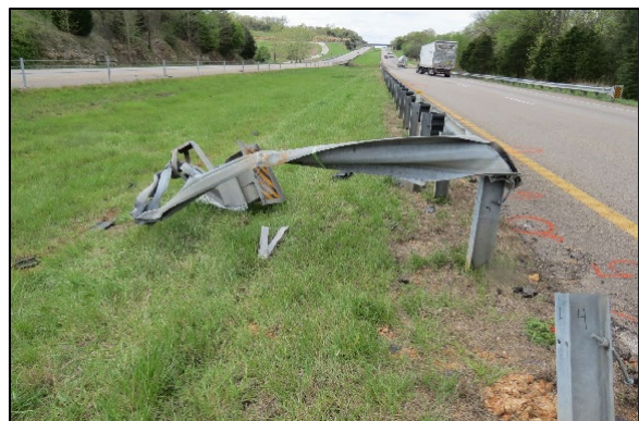
Figure 6: The damaged End terminal and guardrail (guardrail moved post-crash), view northwest
