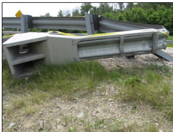
Figure 7: East facing side view depicting the location of the displaced end terminal.
