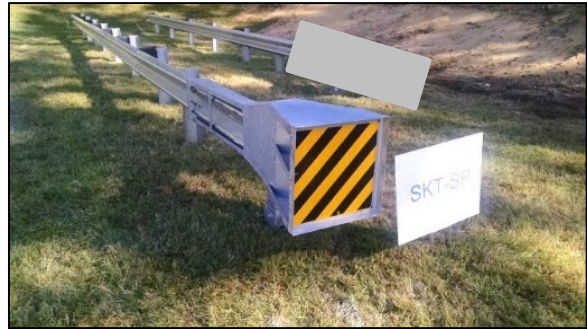
Figure 5: Image depicting an exemplar SKT installation.
