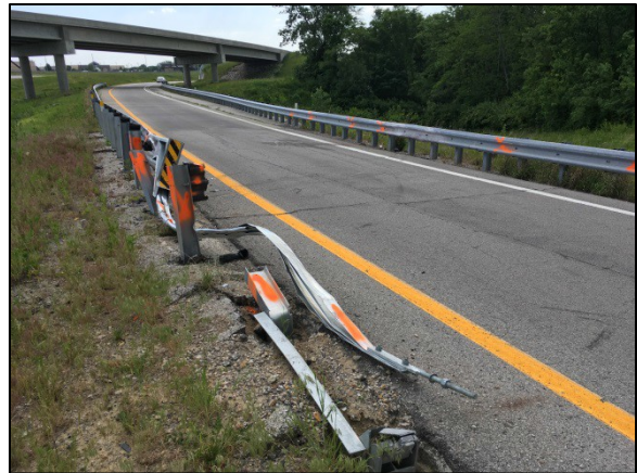
Figure 10: West-looking image of the guardrail at its initial inspection by the MoDOT inspector. Image supplied by MoDOT.
