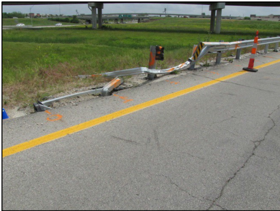
Figure 9: South-looking oblique view of the deformed guardrail system at the SCI inspection.
