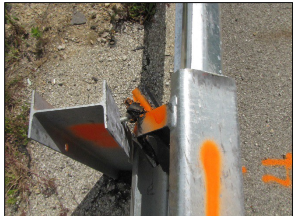
Figure 12: Overhead view of the downstream aspect of the end terminal depicting its capture on the Post 4 carriage bolt.
