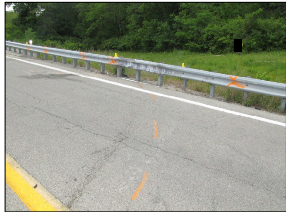
Figure 5: Southwest-looking trajectory view toward Event 2 impact with the face of the guardrail on the opposite roadside.
