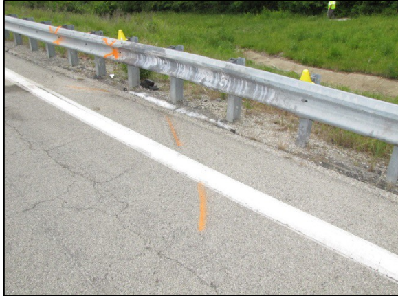
Figure 6: Southwest-looking image depicting the guardrail impact of the opposite road side.
