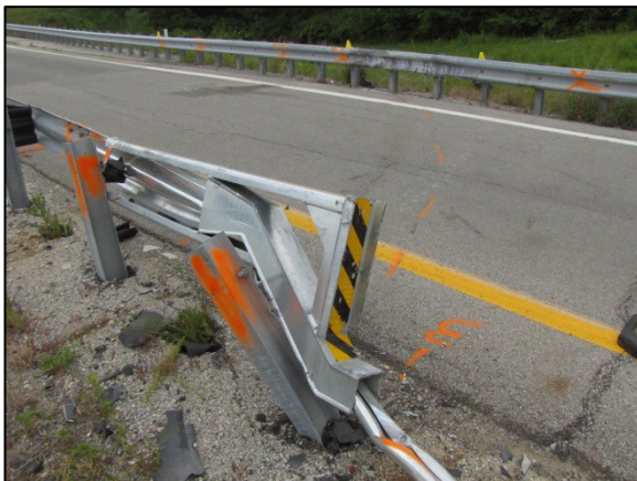
Figure 11: Northwest-looking oblique view of the displaced end terminal.
