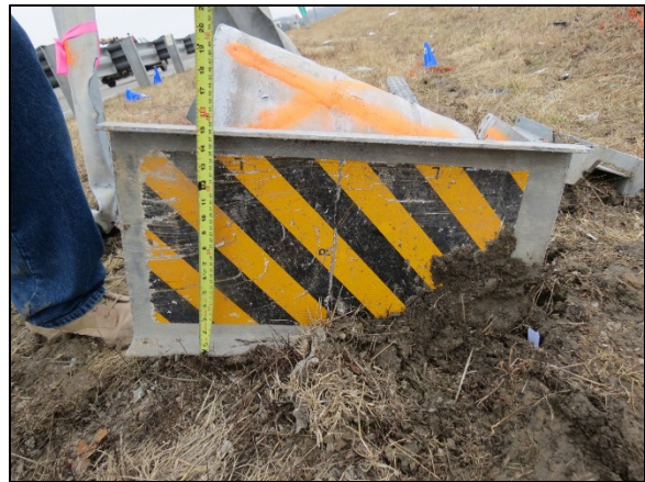
Figure 5: The damaged ET-Plus.
