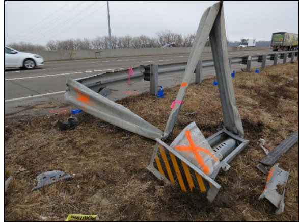
Figure 1: The damaged ET-Plus and guardrail.
