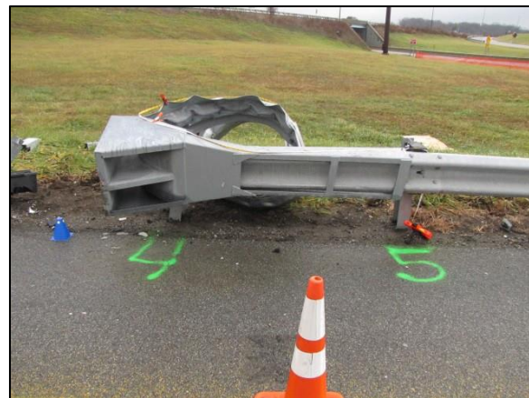
Figure 8: Side view of the location of the displaced end terminal.
