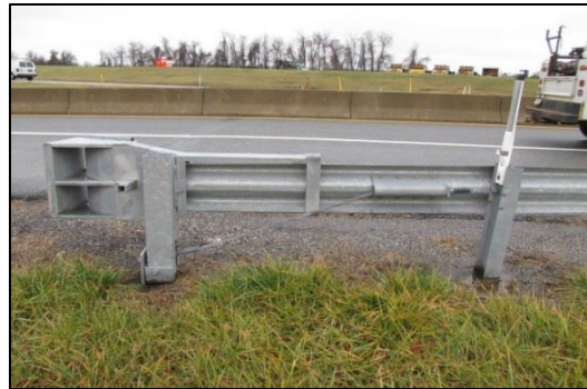
Figure 6: Image showing an exemplar SKT installation.
