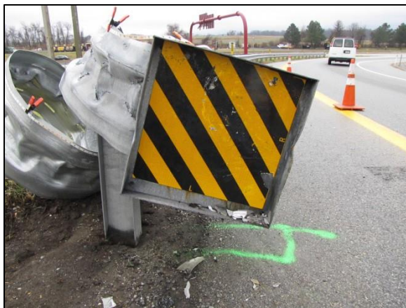
Figure 7: Image showing the struck end terminal and the extruded W-beam.
