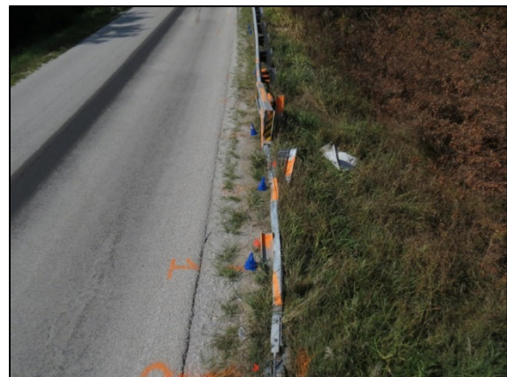
Figure 7. Trinity SoftStop guardrail end terminal, looking west
