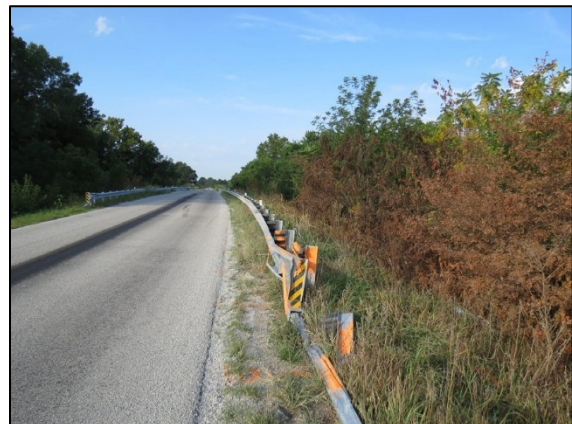
Figure 4. Guardrail end treatment impact
