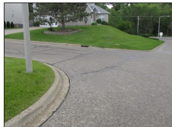
Figure 3: Northwesterly view of the struck landscape wall and the rollaway trajectory of the Dodge.
