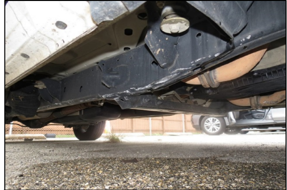
Figure 9. Undercarriage damage (right frame rail), 2014 Ram 1500.
