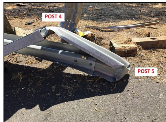
Figure 8. On-scene image, kinks in W-beam at posts 4-5 (police department photo).
