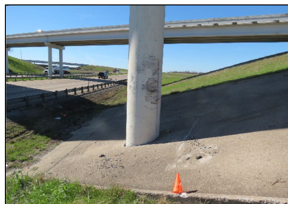
Figure 6: Impact with concrete bridge support pillar looking west
