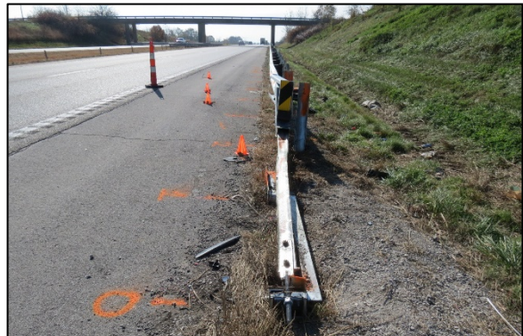
Figure 1. The damaged end terminal and guardrail, view south.
