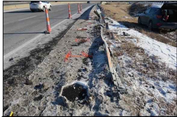
Figure 1: The damaged guardrail and end terminal, view northeast
