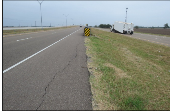
Figure 4: Southbound approach to impact with React 350 crash cushion
