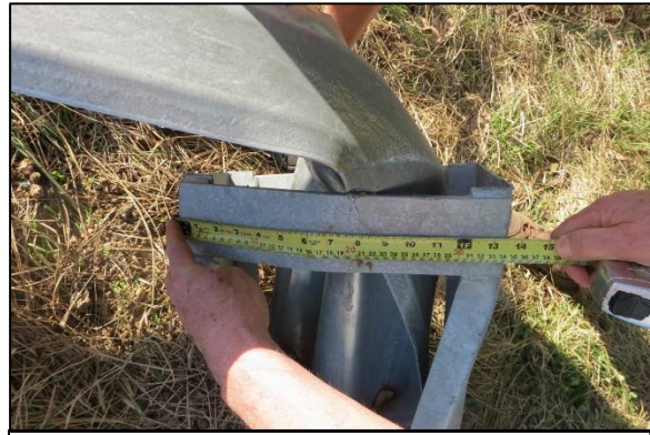
Figure 10: Twisted guardrail at the entrance to the feeder channel
