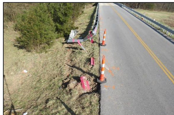
Figure 9: View east to the damaged and displaced posts and guardrail
