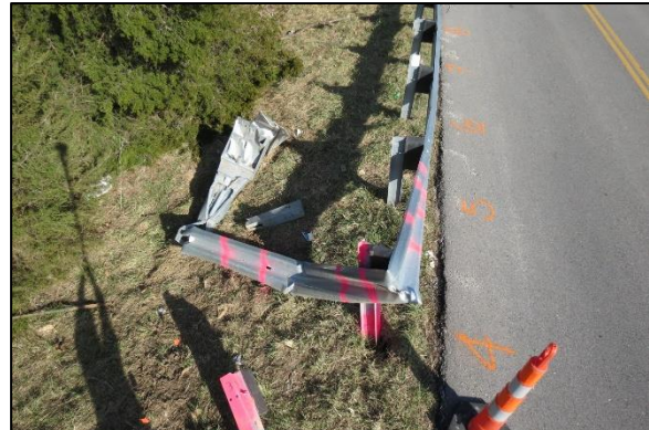
Figure 1: Overhead view of the damaged end terminal and guardrail
