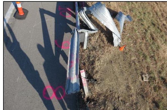
Figure 6. Kinks in the damaged guardrail.
