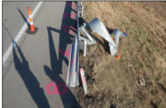
Figure 1. The damaged ET-Plus and guardrail.
