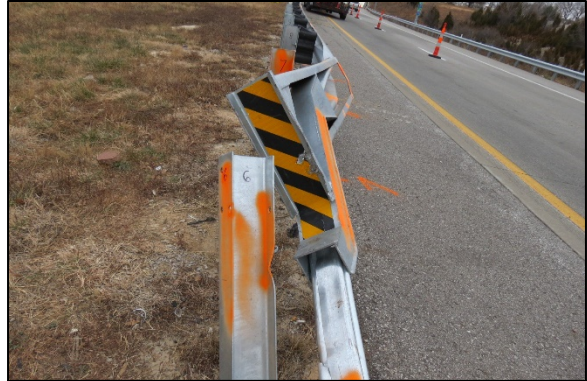
Figure 4. The damaged Soft Stop end terminal, view north.
