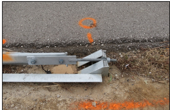
Figure 5. Post zero with anchoring bolt intact.
