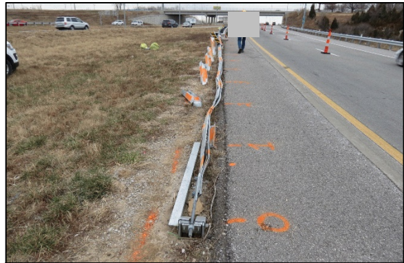
Figure 1. The damaged guardrail, view north.
