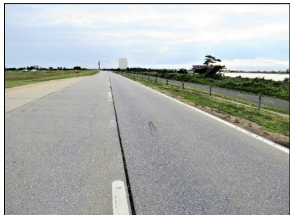
Figure 4. West-facing view of the area of impact in the left aspect of the right travel lane.
