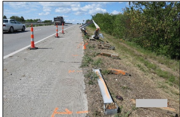
Figure 2. The damaged posts and guardrail, view north.
