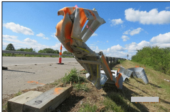
Figure 8. Kinks in guardrail, view north.
