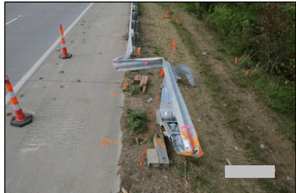
Figure 1. The damaged ET-Plus and guardrail.
