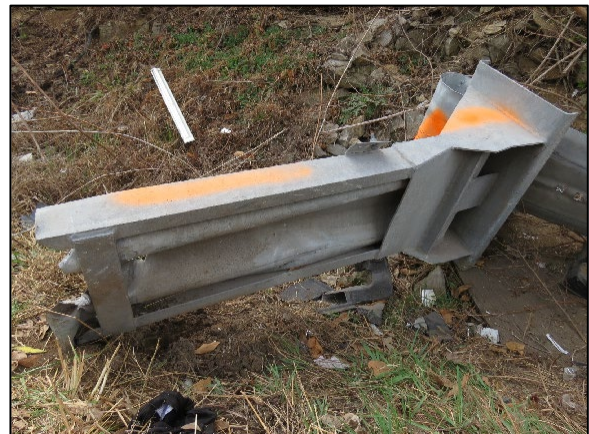
Figure 4. The damaged end terminal.
