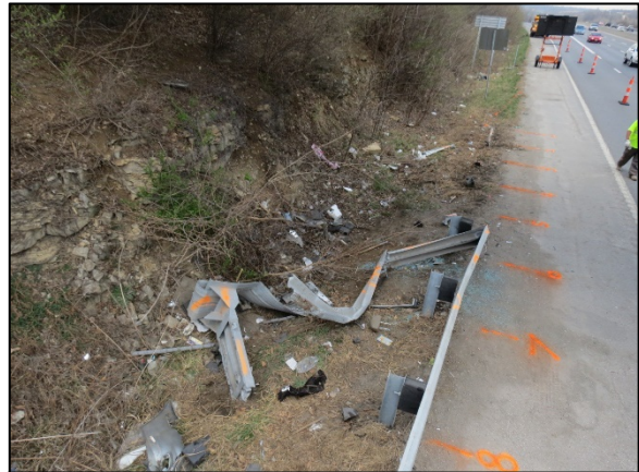
Figure 1. View north to the damaged end terminal and guardrail.
