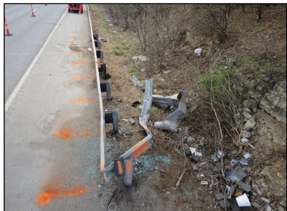
Figure 9. The kinked sections of guardrail, view south.
