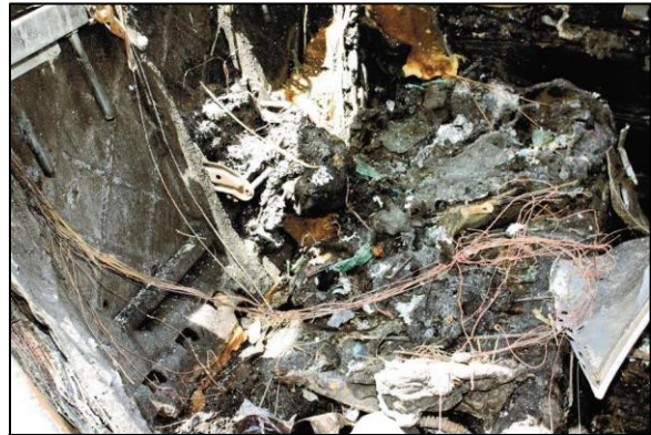
Figure 7. Fire damage to the front row of the BMW. (Image obtained from an online VIN source.)
