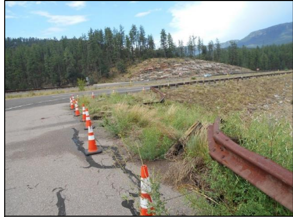
Figure 3. Guardrail impact, looking north (police image).
