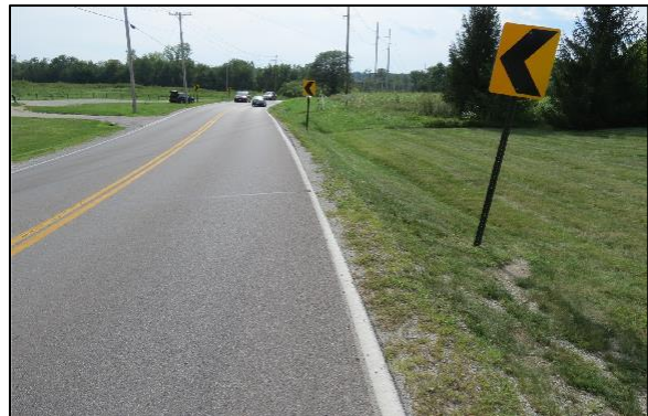
Figure 3: Westbound view of the area of roadway departure and approach to impact with two chevron alignment signs.
