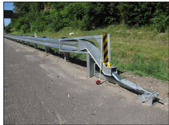
Figure 8. Image depicting an exemplar Soft Stop end terminal and guardrail located approximately 18 km (11 miles) west of the crash site.
