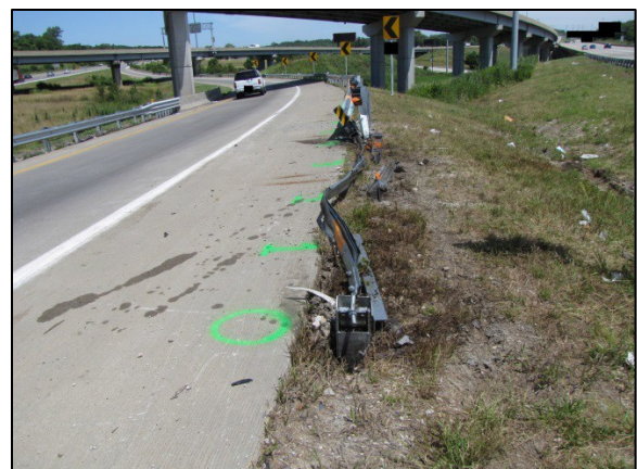
Figure 6. North-facing trajectory view of the Ford at impact with the guardrail.
