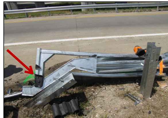
Figure 11. West-facing image depicting the location and condition of the displaced end terminal adjacent to posts 4 and 5.
