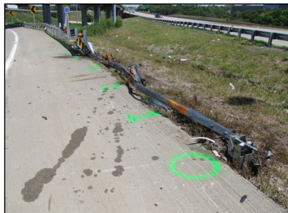
Figure 3. North-facing view of the crash site and the damaged guardrail during the SCI inspection.
