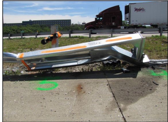
Figure 10. East-facing image depicting the location and condition of the displaced end terminal adjacent to posts 4 and 5.
