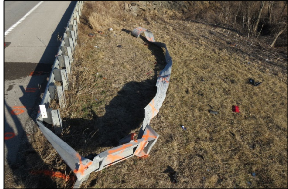
Figure 1. The damaged end terminal and guardrail.
