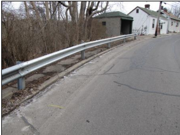
Figure 3: Northerly view of the struck (and replaced) W-beam guardrail system.
